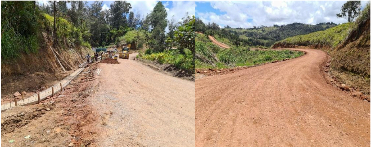
Photo 69: Pavement stabilization, bituminous surfacing and associated works of Meraimanda-Birip (16.5km) on Wabag-Kompiam Road
