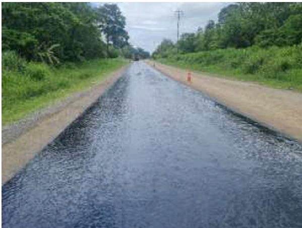
Photo 16: Yakumbu Bridge Reconstruction, Priming and Sealing of a Section on Ramu Highway
