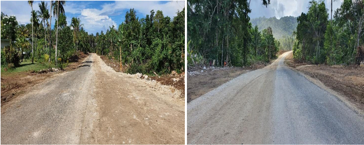
Photo 11: Road Widening and Pavement works on West Coast Road, New Ireland Province
