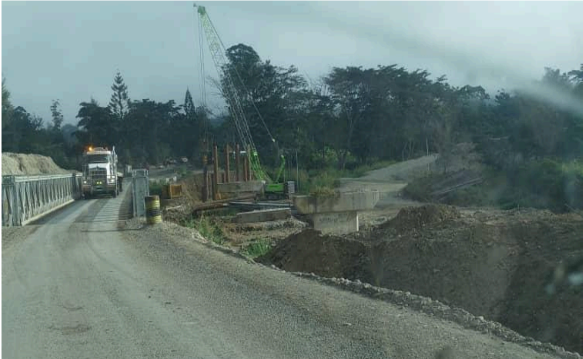
Photo 58: Replacement works on the Bena Bridge, Highlands Highway under SHHIP Tranche 2 to 4-Lane Bridge.
