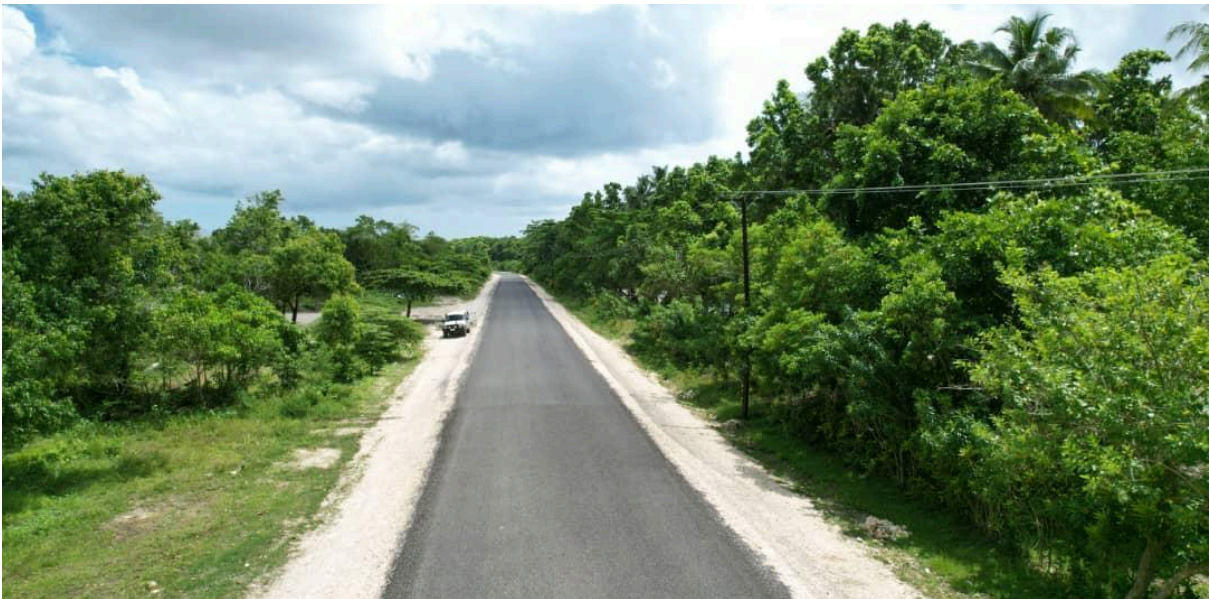
Photo 29: Resealing Works on going along Boluminski Highway under Long Term Maintenance Contract.
