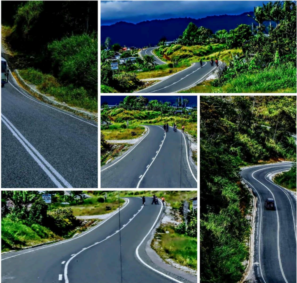
Photo 23: Upgrading and Sealing Works of the Kagua-Erave Section of the Gulf-Southern Highlands Highway CIVPAC, a local contractor. This Highway is expected to be completed by 2026.
