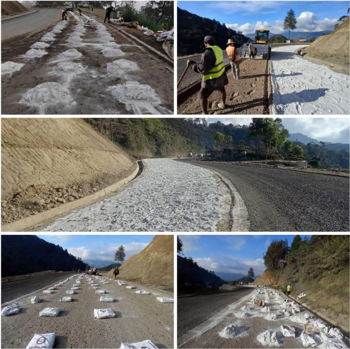
Photo 48: Upgrading, Stabilization and Asphaltting of the notorious unstable Daulo Pass Section of the Highlands Highway with the latest stabilization and asphaltting standards to achieve reliability and climate resilience surface.
