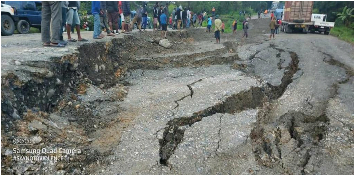
Photos 103: Another example of a Road Section collapsing under the weight of climate Change related natural disaster.
