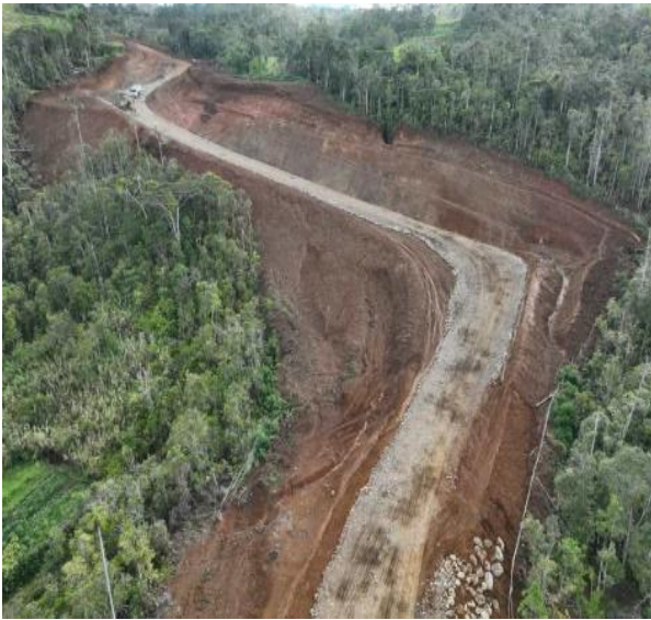
Photo 39: Construction of Pilot Track from Piribu to Angore, Hela Province, under Exxon Mobil
