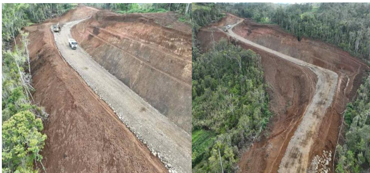
Photo 65: Construction of Pilot Track from Piribu to Angore, Hela Province, under Exxon Mobil
