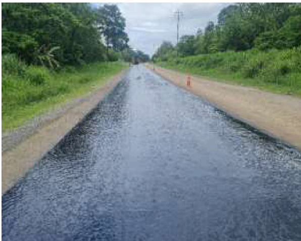
Photo 45: Yakumbu Bridge Reconstruction and Priming and Sealing of a Section on Ramu Highway
