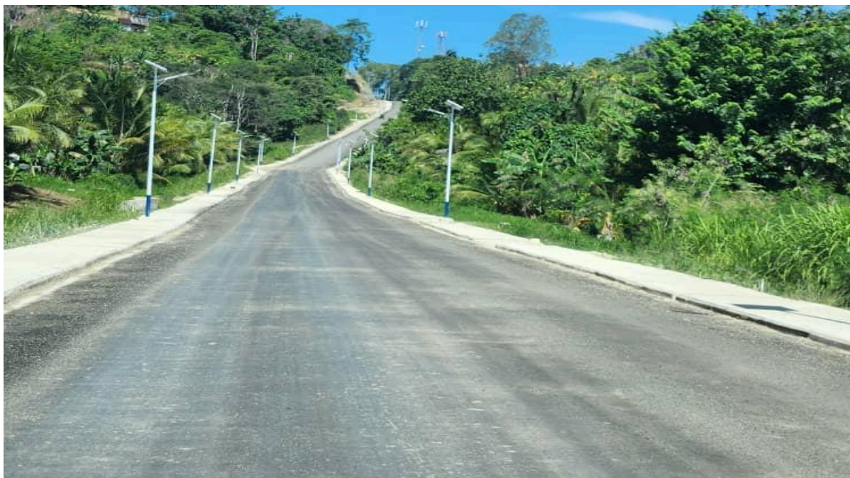
Photo 46: Recently upgraded Section of the Sepik Coastal Highway -Sandaun Province, that will support PNG-Indonesia Border Trade.
